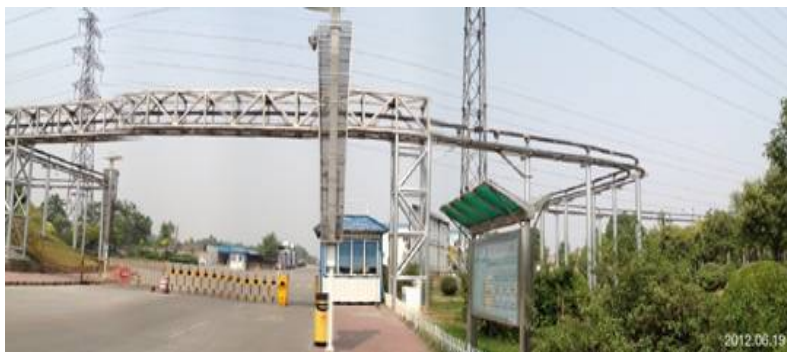
Fig. 3 An overview of the 10kA HTS DC power cable after installation.
