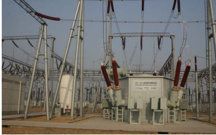
Fig. 4 A view of the 220kV/800A FCL after installation at Shigezhuang substation in Tianjin
