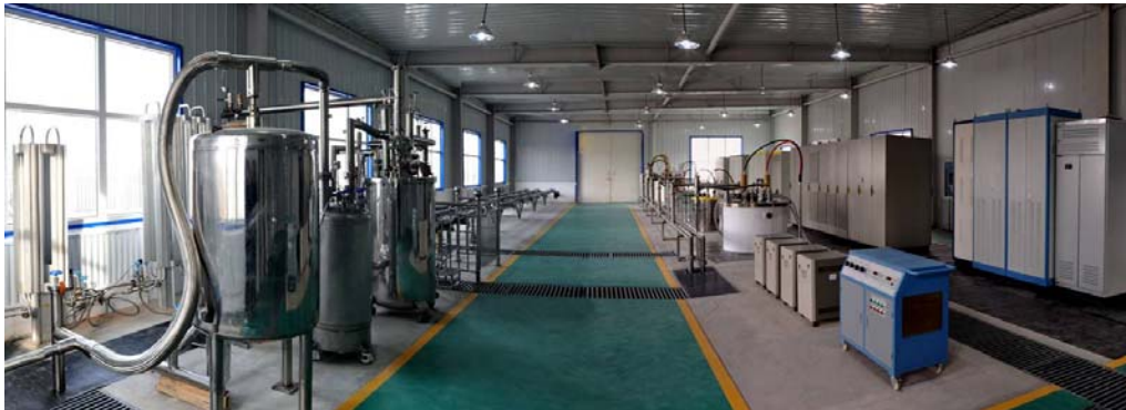
Fig. 2 A view of the superconducting power substation
