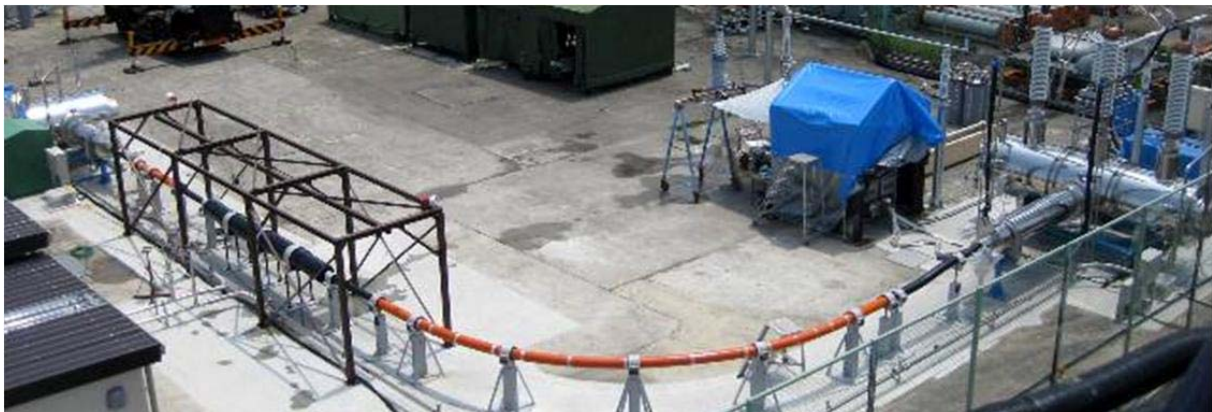
A 30 m HTS cable system for pre-verification
