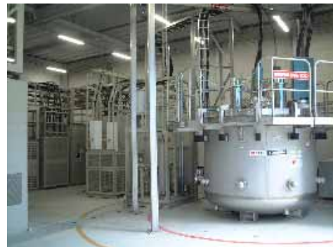
Fig.1 5 MVA - 5 MJ SMES system for bridging instantaneous voltage dips
